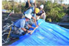
Contractors install roofing material for Project Blue Roof in this Florida photo from the Army Corps of Engineers. Emergency recovery programs such as this could suffer under a suggestion that Trump use the money for his proposed border wall.
